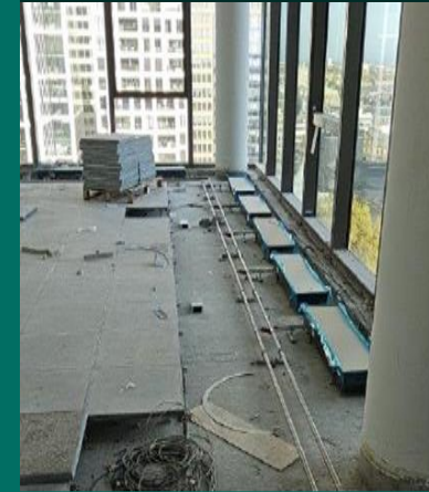
Mechanical and electrical works below raised floor
